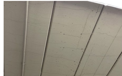
Figure 7: Underside of a cracked RAAC panel
