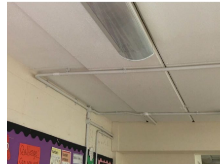
Figure 10: Example of deflected RAAC panel
