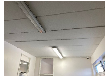
Figure 11: Example of deflected RAAC panel
