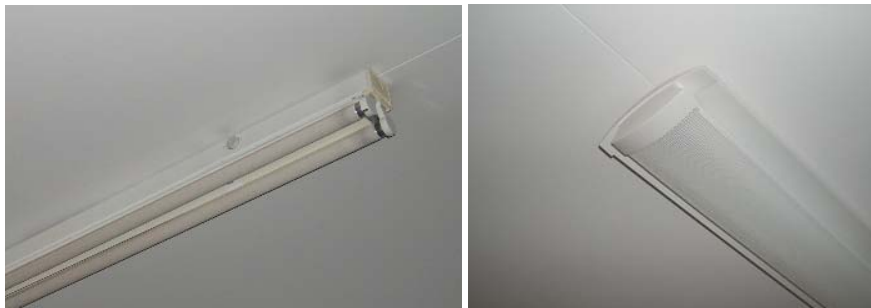
Figure 3.4 Upgrade of lighting fitting.
